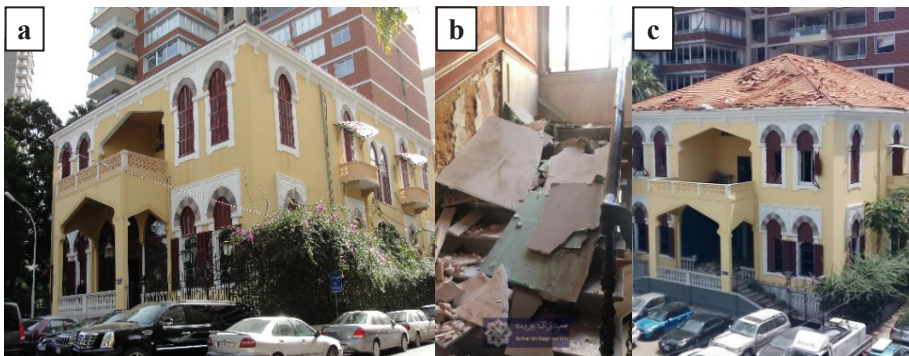
Fig. 19: Villa Linda Sursock before the explosion (Bilgili, 2018), b: Villa Linda Sursock interior damages explosion (BeirutHeritageSociety, 2020), c: Villa Linda Sursock's exterior damage after explosion (BeirutHeritageSociety., 2020).
