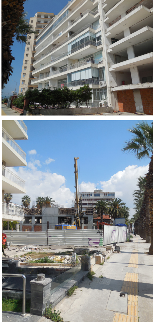
Figure 3.6. Apartments Waiting to Be Demolished and Being Rebuilt due to Impact of the 2020 Earthquake in Karşıyaka Coast (Eti Akyüz Levi Archive -2023)
