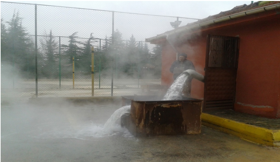
Photograph 2: Temperature and Flow Measurement in a Newly Opened Well in Karacasu
